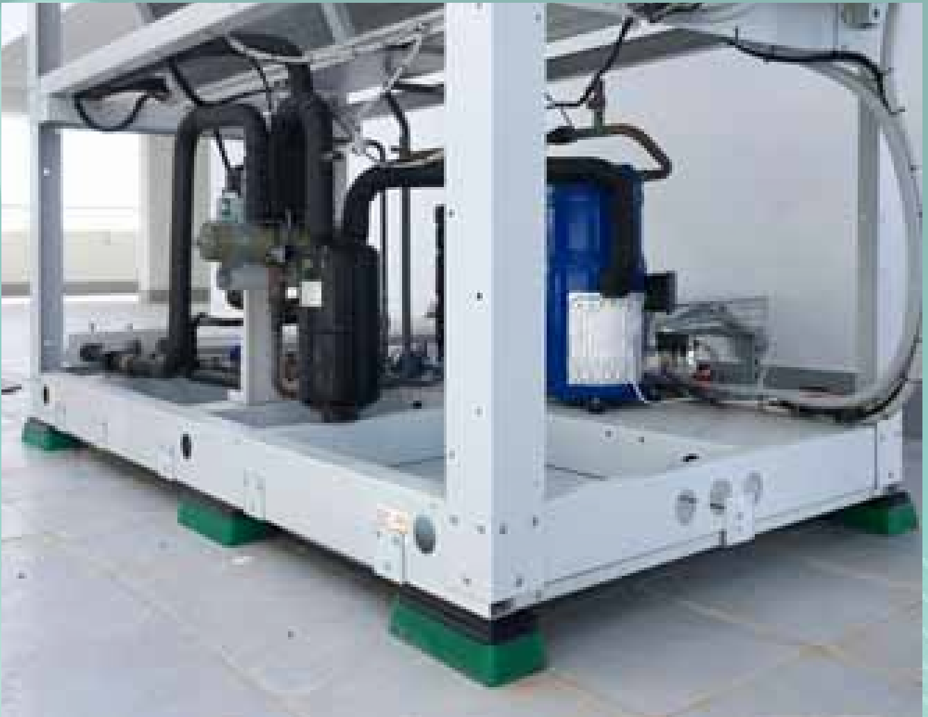
Arco Green Damping - heat pump
